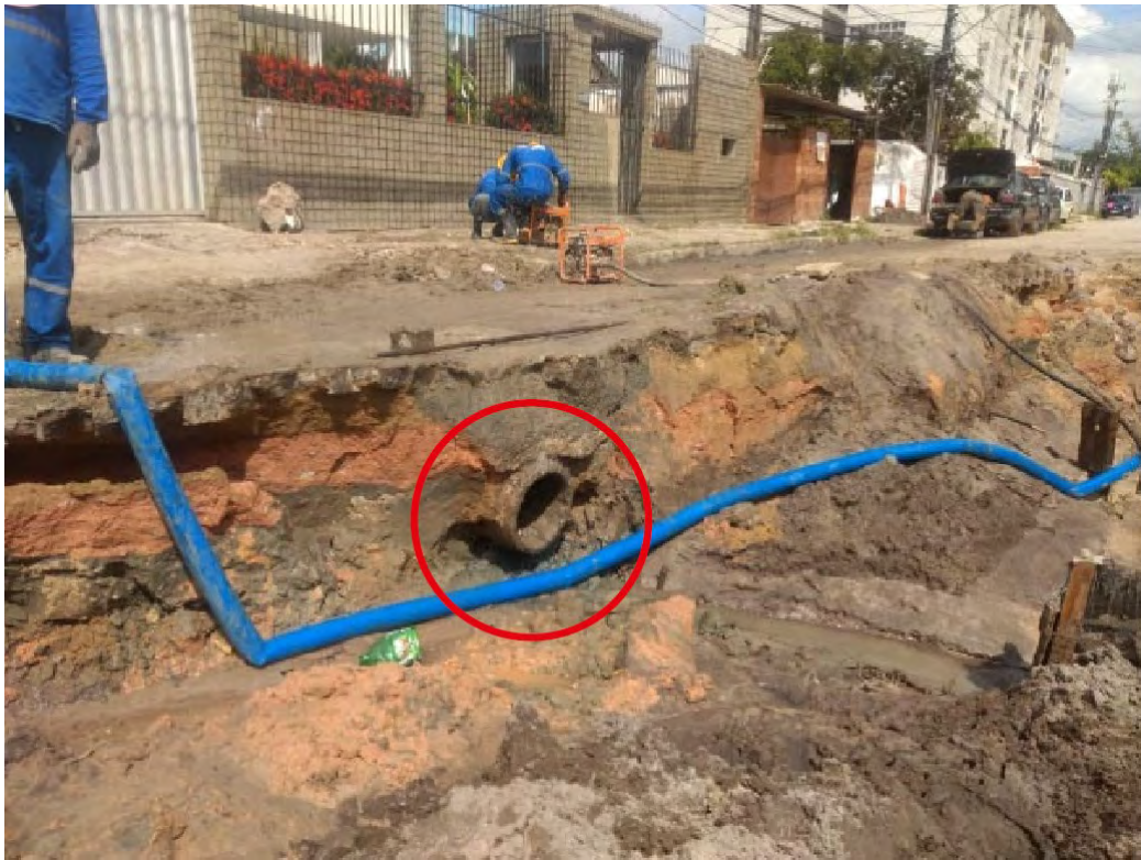
Figure 3 When executing the collector, deactivated drainage networks were found at Rua Feliciano Lins, Recife.
