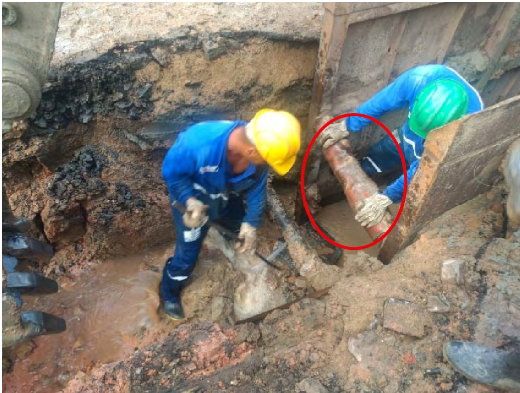
Figure 1 Damage to the drainage network, at Rua Feliciano Lins, Recife during excavation for the construction of Collector.
