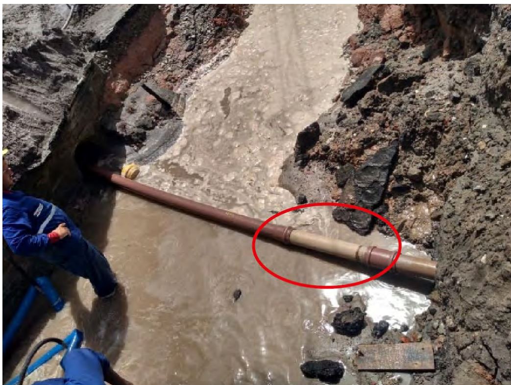
Figure 2 Damage to the drainage network, at Rua Feliciano Lins, Recife during excavation for the execution of Collector.
