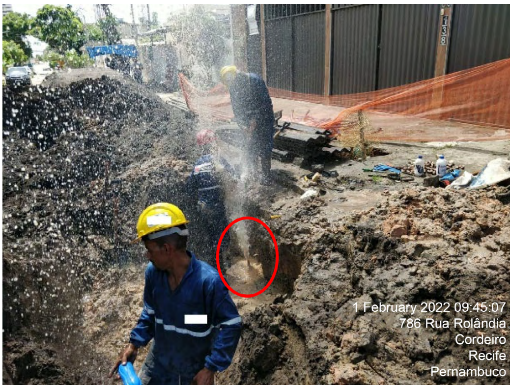
Figure 4 When carrying out the extension, drainage networks were found, on Rua Rolândia, Recife.
