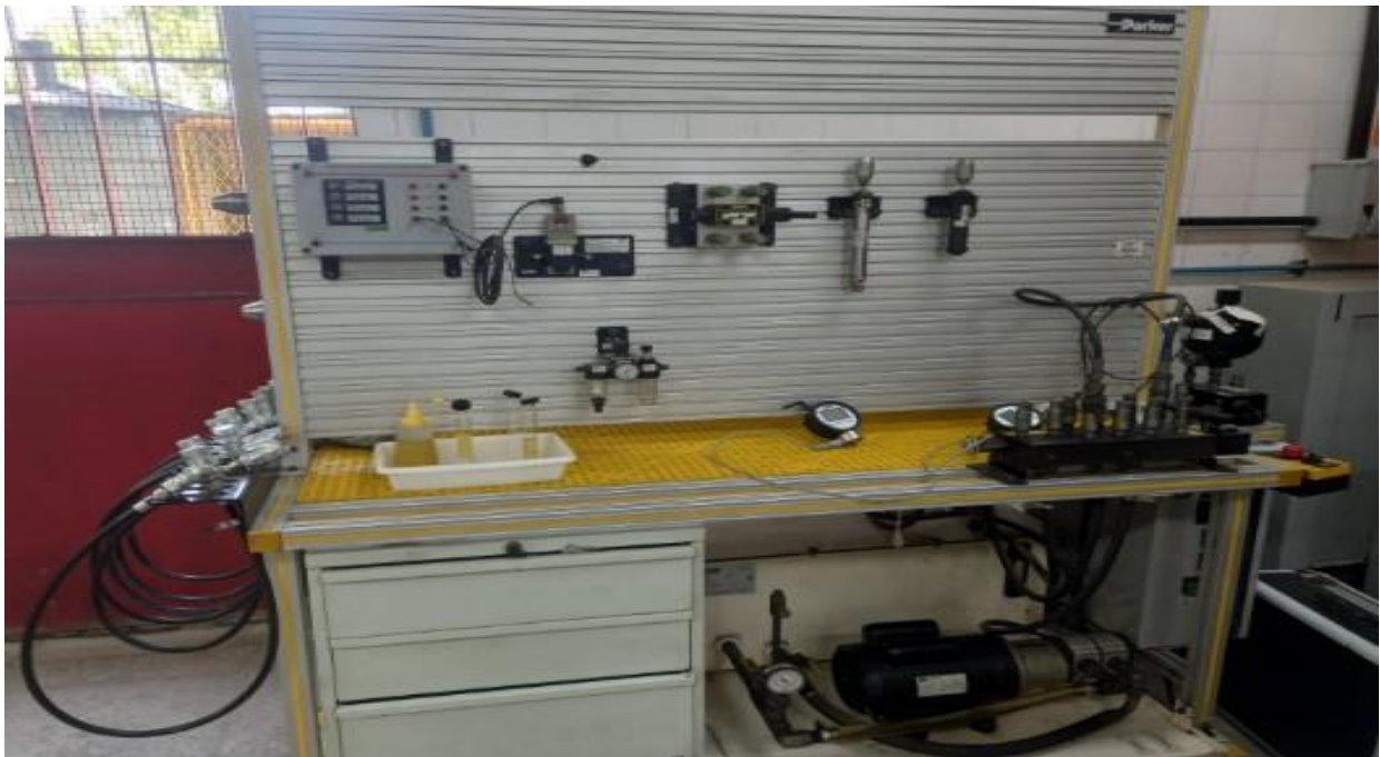
Figure 1. HDP Pneumatic and Hydraulic Module Equipment in the Industrial Processes Laboratory.
