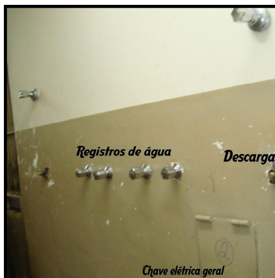
Image 1 - Control access to water and electricity
