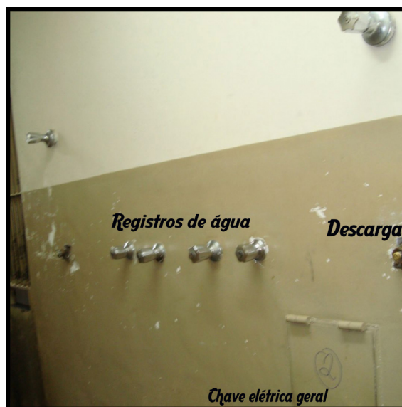
Image 1 - Control access to water and electricity
