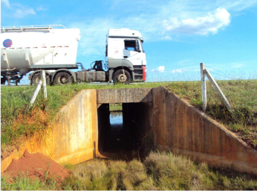
Figure 3. An example of a box culvert under a highway evaluated for the cost-benefit analyses (Copyright © 2012, by Fernanda D. Abra). Note that this particular culvert measures 2.00x2.00m and that we evaluated a culvert that is 3.00x3.00m.
