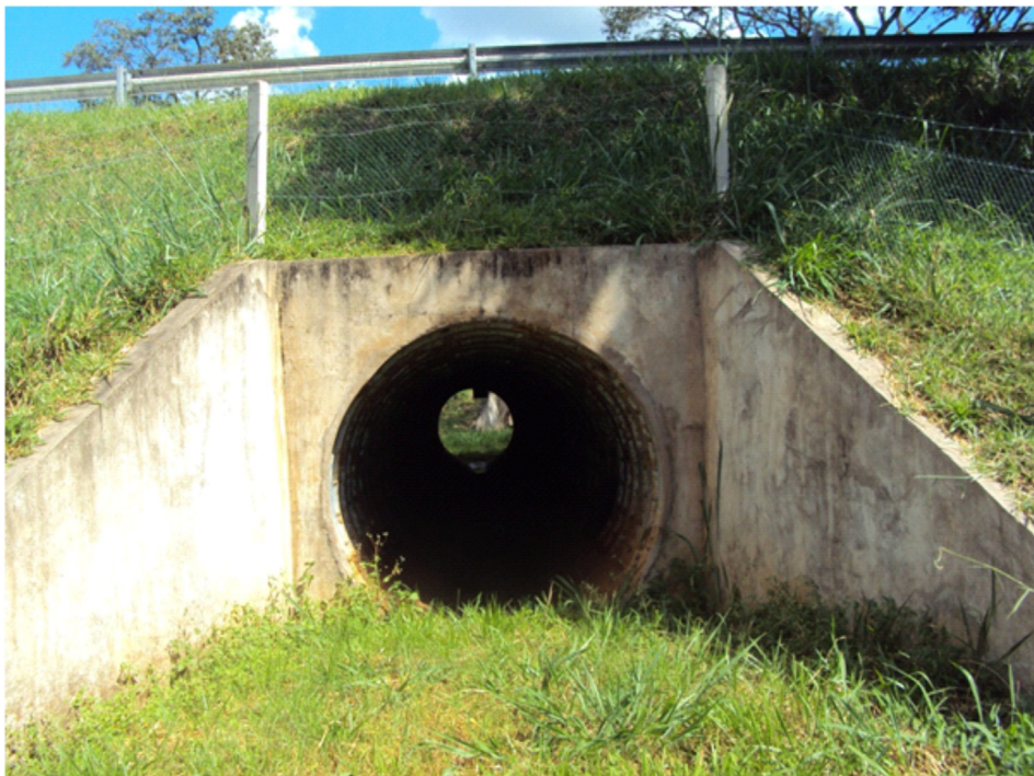
Figure 2. An example of a 1.7m diameter culvert under a highway evaluated for the cost-benefit analyses (Copyright © 2012, by Fernanda D. Abra).
