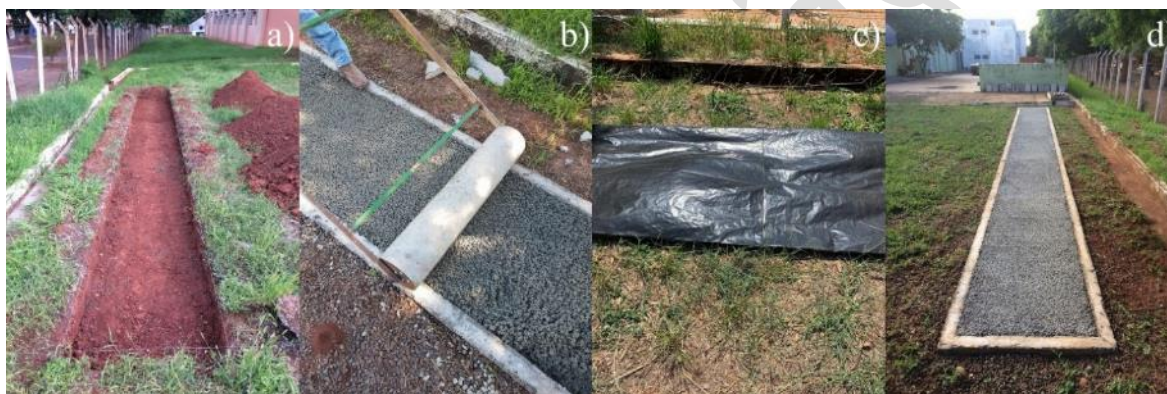
Figure 5: Stages of pavement construction: (a) Excavation; (b) Placement, consolidation and finishing; (c) Curing procedure; (d) Finished pavement
