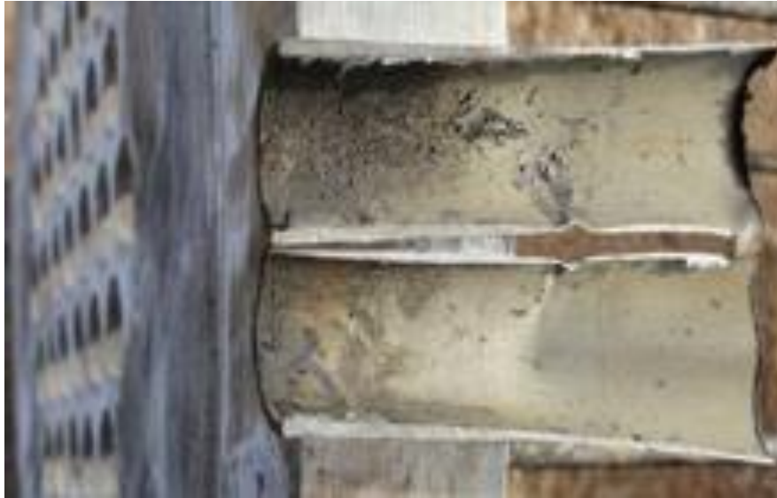
Figure 8: Corrosion in a shell and a SAF-2507 tube heat exchanger which raises the temperature of glycerin to 95°C.
