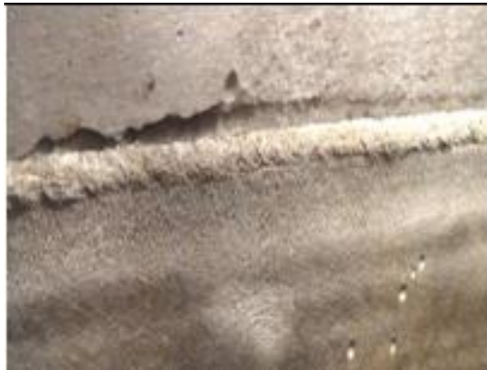
Figure 7: Corrosion in a cylindrical decanter vessel in the lower generators of the vessel, especially in the regions adjacent to the assembly welds.
